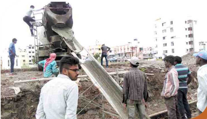
Emerging as a Structural Engineer
